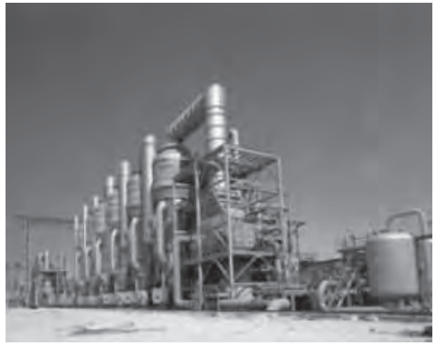
Desalination plant, capacity - 120,000 m 3 of fresh water per day
